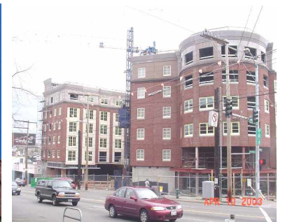
Silver Cloud Inn, Seattle, WA, USA, curved full height and spandrel panels
